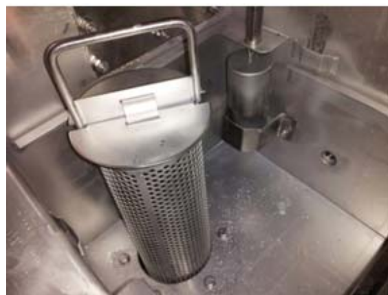
Pump filter in drain sump
