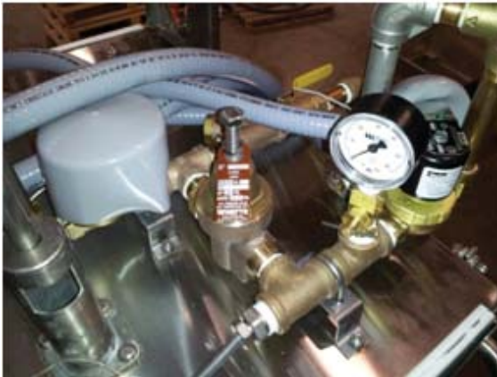
Showing PRV, ASSE approved air-gap, final rinse gauge
