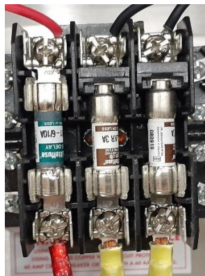
44 3ph transformer, left fuse 1a
