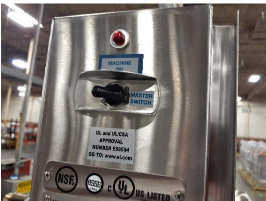
Master switch with control light above
