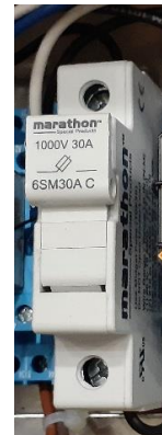
All other control fuses, 10a
