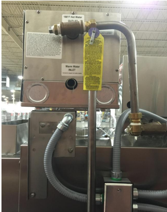
Inlet of the booster is 62.5" AFF, top of booster is 71" AFF
