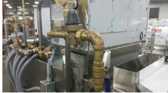
If PRV is required (only if 50psi or above) install here, not supplied
