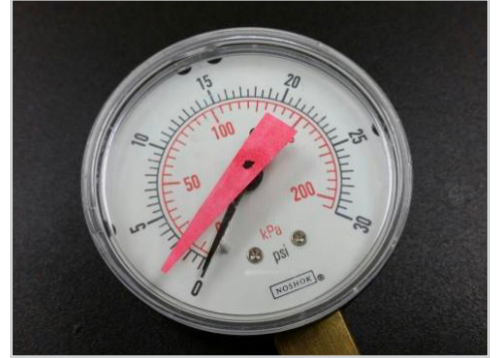
Water Curtain (Pumped Rinse) on conveyor is approx 2-3 psi
