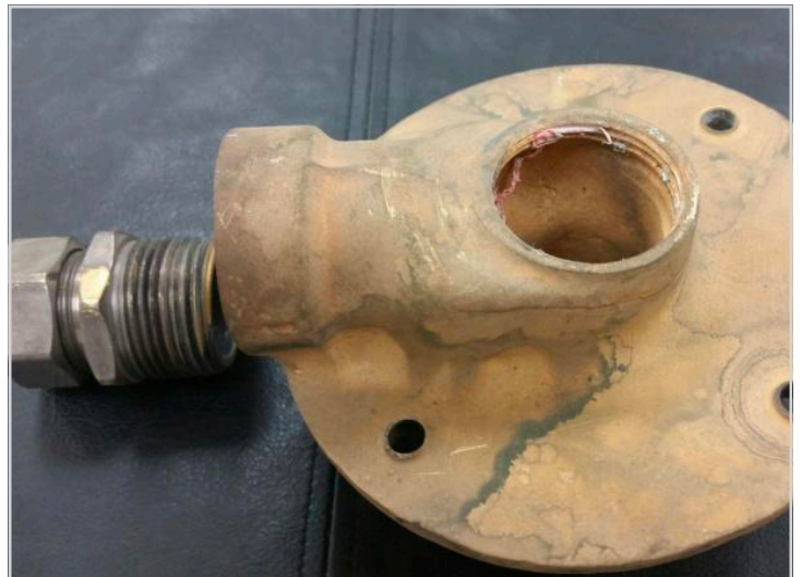
Chemicals erode the base, threads would no longer fit
