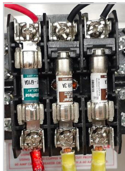
44 3ph transformer, left fuse 1a
