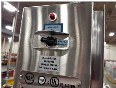
Master switch with control light above
