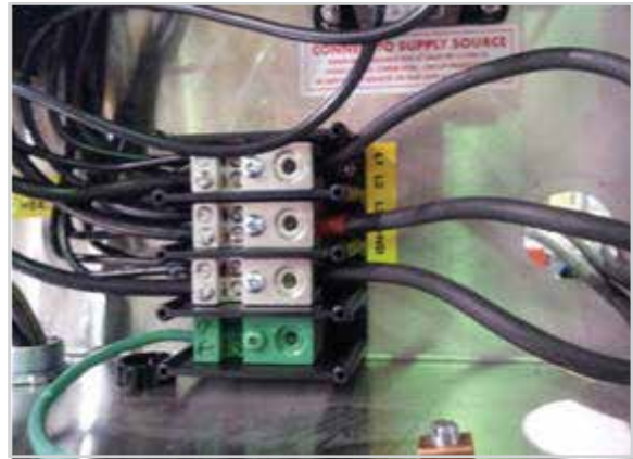
Main distribution block for 44's incoming 3-phase
