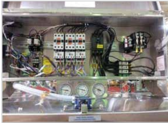
ADC-44 conveyor control box for 3-phase power
