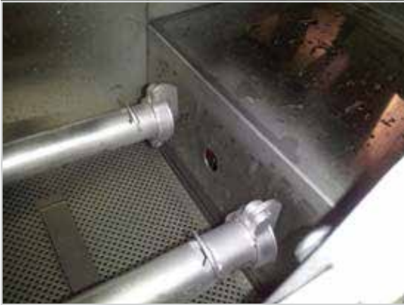
Showing hole at the side of tank, 7/8" detergent fitting
