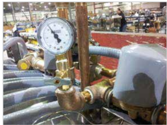
Final rinse manifold with pressure gauge, 20 psi flow req.
