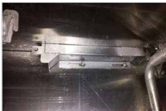
Showing diverter slide to fill both tanks
