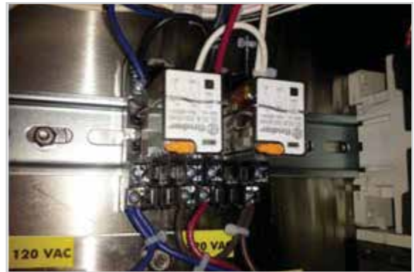
Conveyor motor control relays
