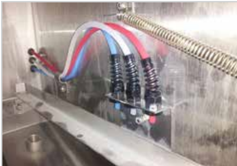
Showing chemical lines above sump
