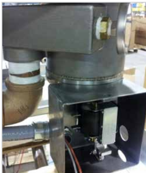
Showing drain solenoid
