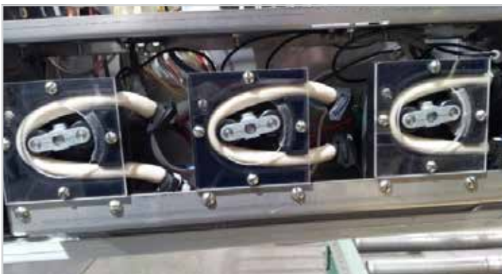
Showing deter, rinse, sanitizer internal chemical pumps
