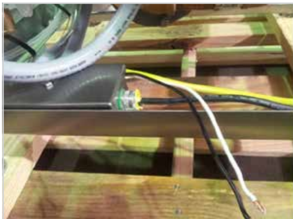
Power junction box for incoming 120v power
