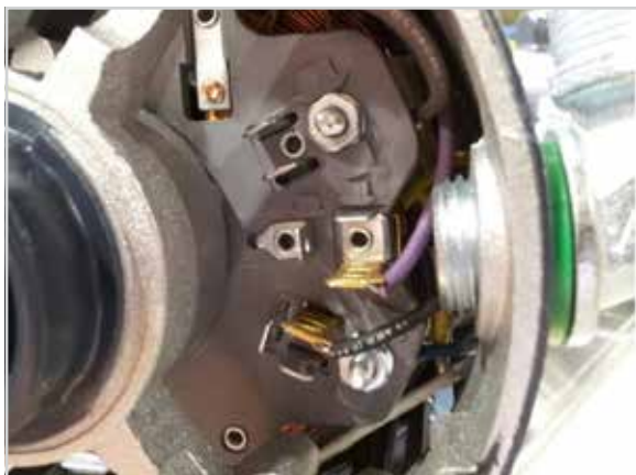
1.5 HP Motor, arrow 1 arrow 2 point to L1 and Neutral connect points
