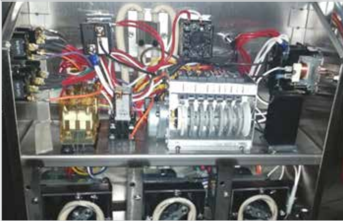
Showing deter, rinse, sanitizer internal chemical pumps
