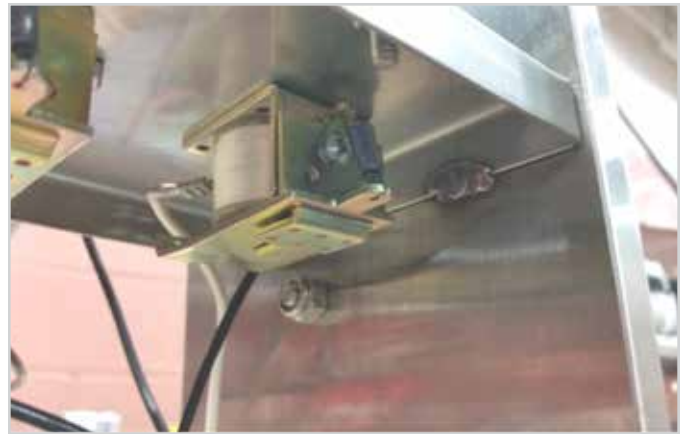
Optional buzzer for low chem alarm, under rack counter
