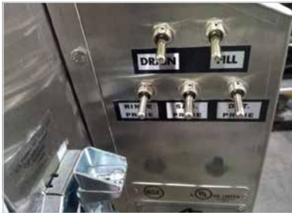
Showing controls on lower access door
