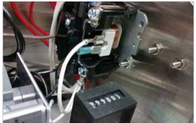
Wash motor contactor next to rack counter
