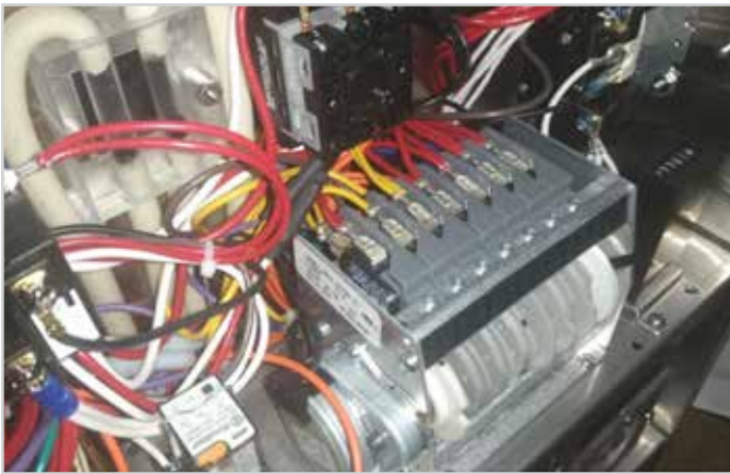
Relays, counter, switches, cam timer, motor contactor
