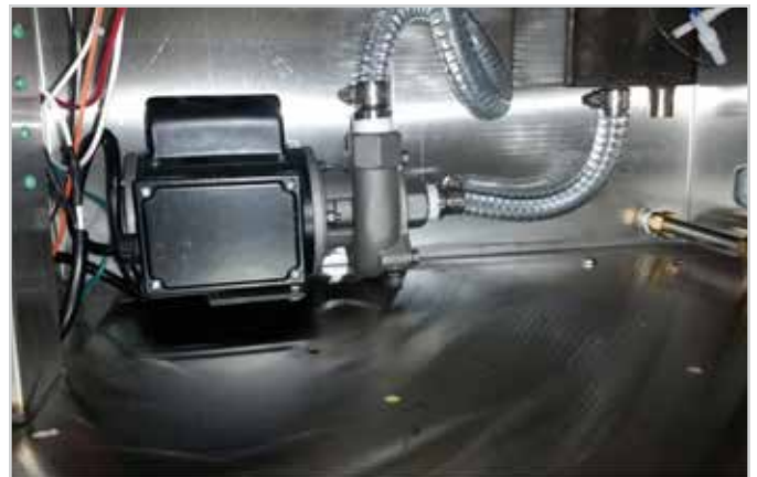
Wash pump with rinse pump removed
