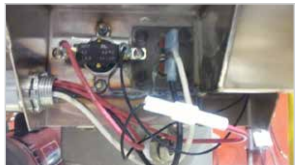
Heater box less cover, thermostat, element, float wires
