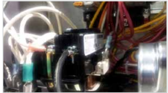
Wash motor contactor to the left of the cam timer motor
