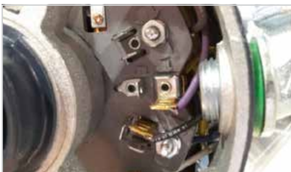
1.5 HP Motor, arrow 1 arrow 2 point to L1 and Neutral connect points
