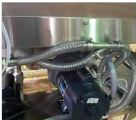
Drain “Y” from overflow & drain pump, 48" drain tube
