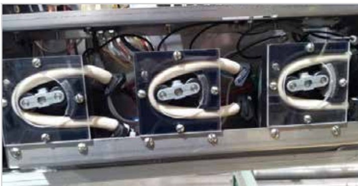
Showing deter, rinse, sanitizer internal chemical pumps
