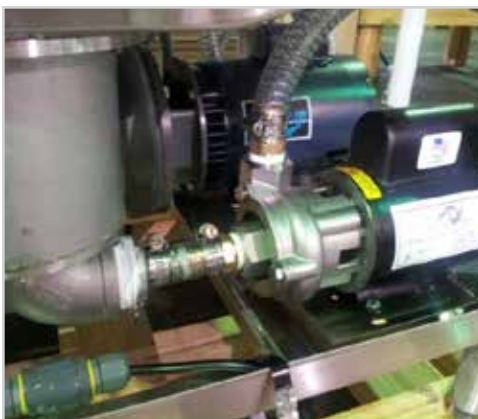
Showing stainless drain pump with 3/4" discharge tube
