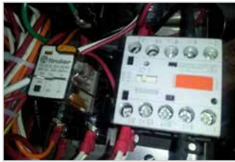
Left is Drain Relay, right is Heater Contactor
