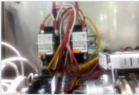
Left is Start Relay, right is Heater Relay
