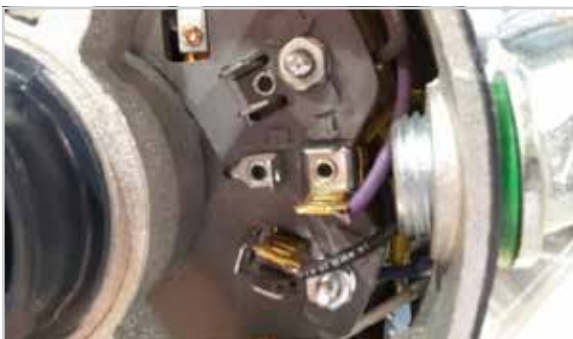
1.5 HP Motor, arrow 1 arrow 2 point to L1 and Neutral connect points
