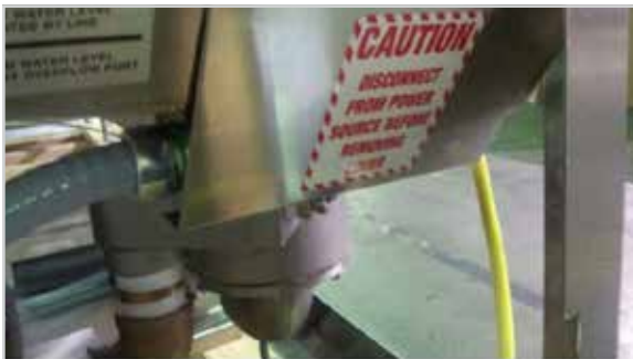
Heater terminal box in right front side of the pan
