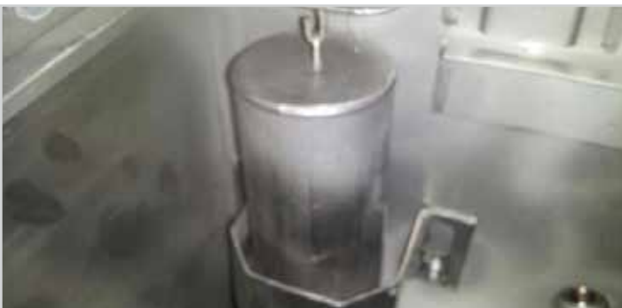
Wash tank float and tank overflow
