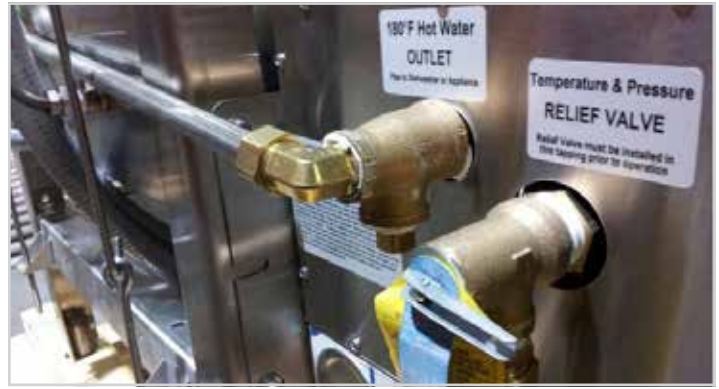
Booster hot outlet line going up to HT-25/34 inlet manifold
