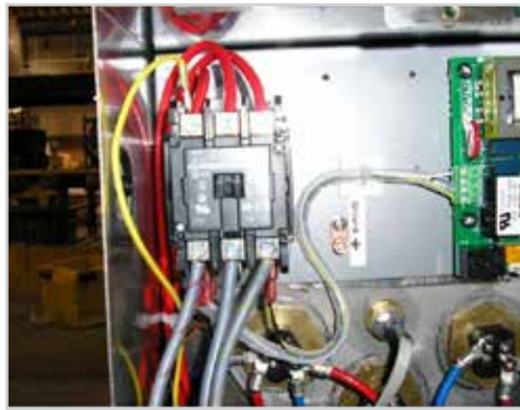
Showing booster contactor, yellow signal wire
