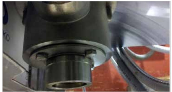
Drain sump connection for copper drain, bottom of tank
