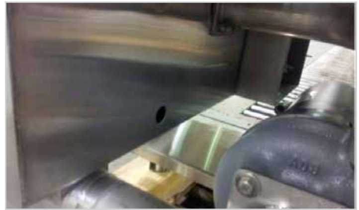
Showing 7/8" detergent probe hole behind pump motor
