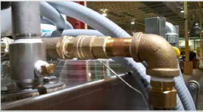
HT hot water inlet ball valve, connected to booster line
