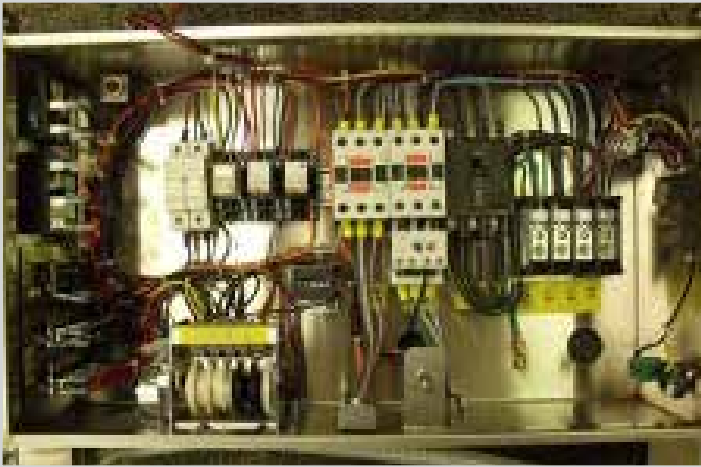
Showing HT-25, 4-wire control box
