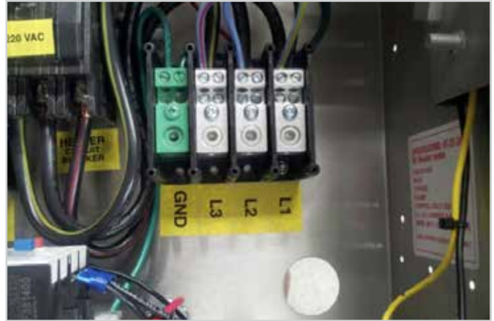
Main distribution block for incoming wire & 1" conduit hole
