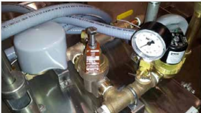
Showing PRV, ASSE approved air-gap, final rinse gauge
