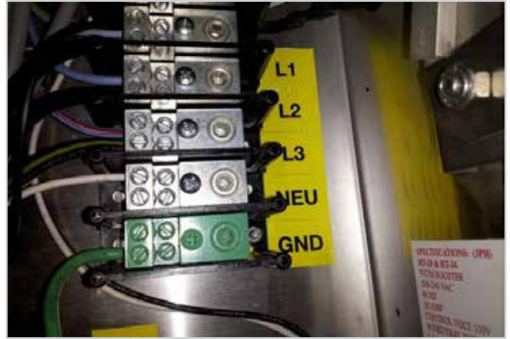
Main distribution block for incoming 5-wire
