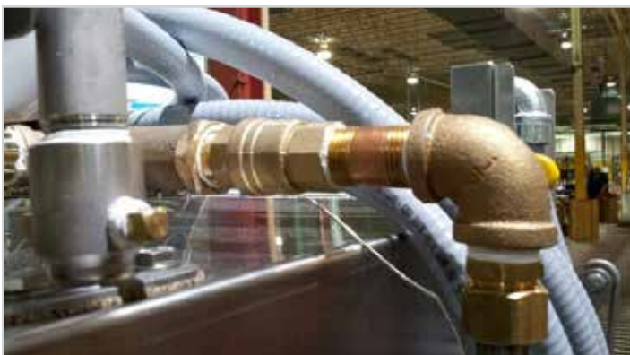
HT hot water inlet ball valve, connected to booster line
