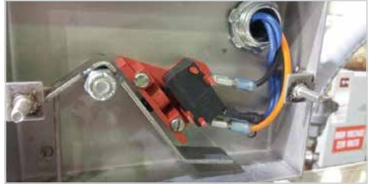
Showing “float” switch that controls fill water & heater
