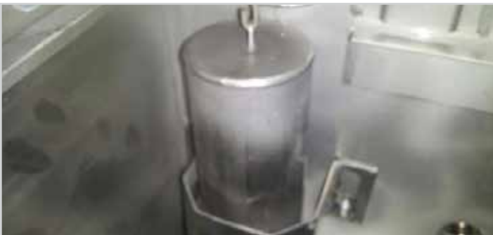
Wash tank float and tank overflow
