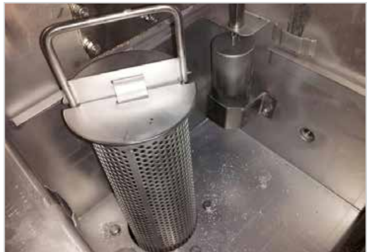
Pump filter in drain sump
