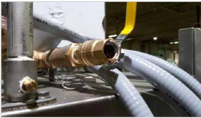
Showing final rinse mixing chamber, hot-water inlet to HT-25
