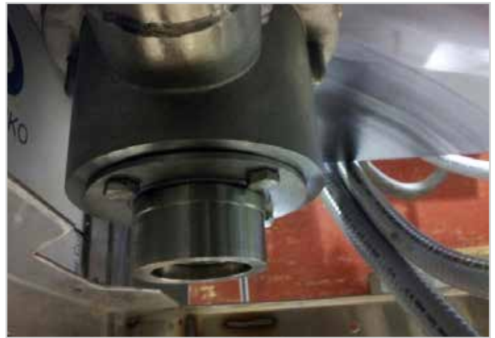
Drain sump connection for copper drain, bottom of tank
