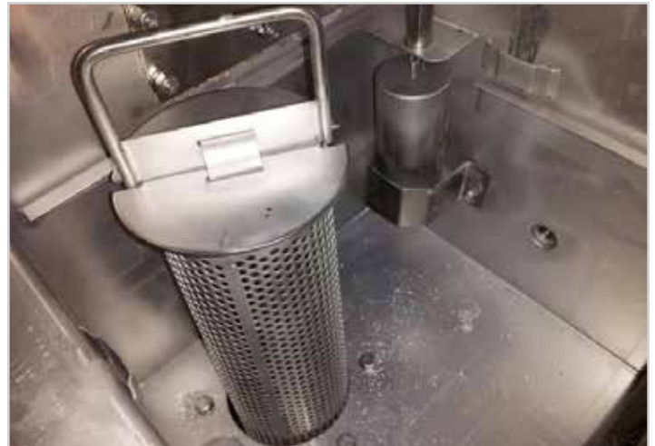
Pump filter in drain sump
