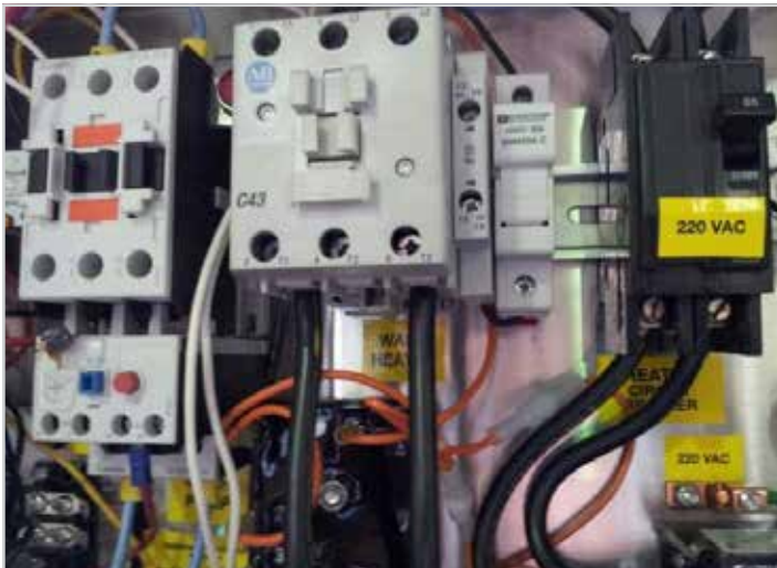
Motor contactor, heater contactor, fuse block, heater breaker
