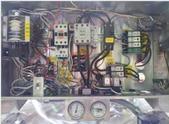
Showing HT-25, single-phase control box
