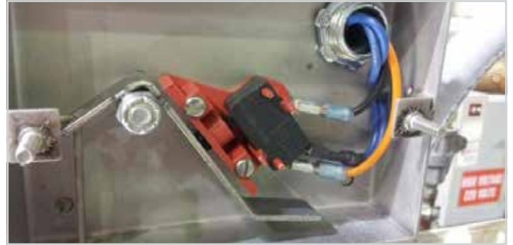
Showing “float” switch that controls fill water & heater
