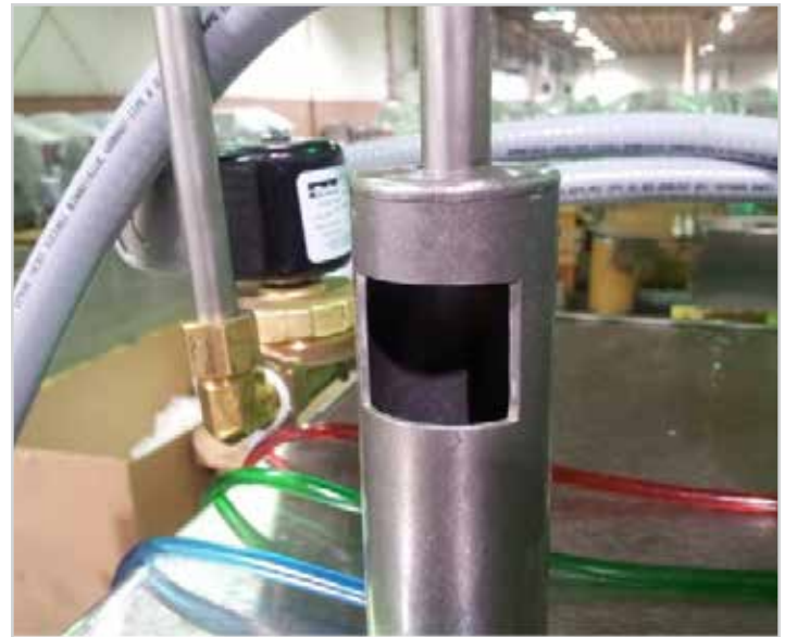
ASSE approved air gap (backflow preventer)
