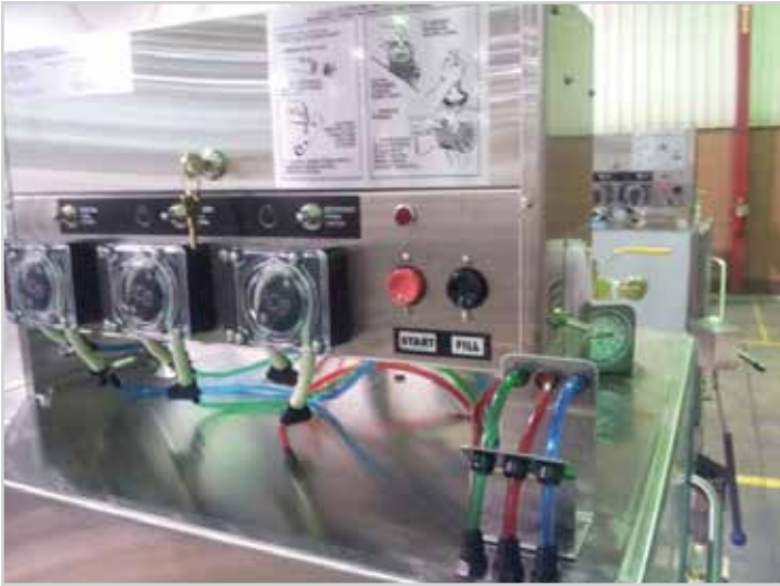
Showing L3DWS control box, chemical pumps, prime switches
