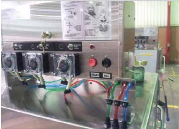
Showing deter, rinse, sanitizer external pumps
