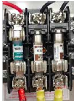
44 3ph transformer, left fuse 1a
