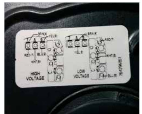
Low voltage is 208-230v, high voltage is 460v
