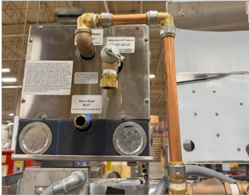
Figure 3. ADC-44 Booster Outlet Tubing
