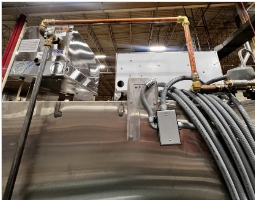
Figure 4. ADC-66 Booster Outlet Tubing
