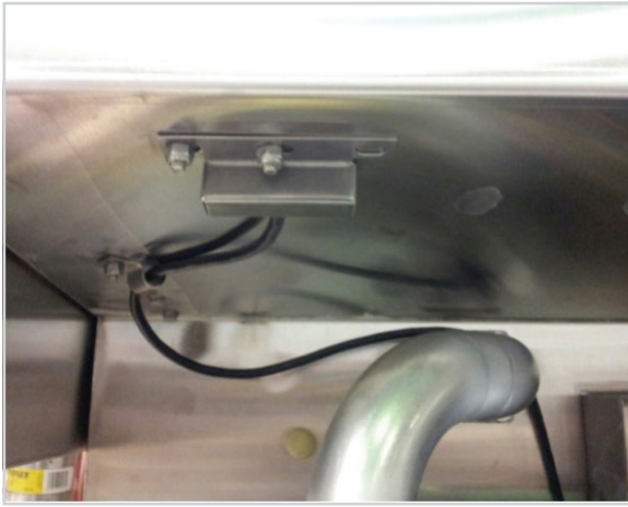
Sequence reed switch for wash tank
