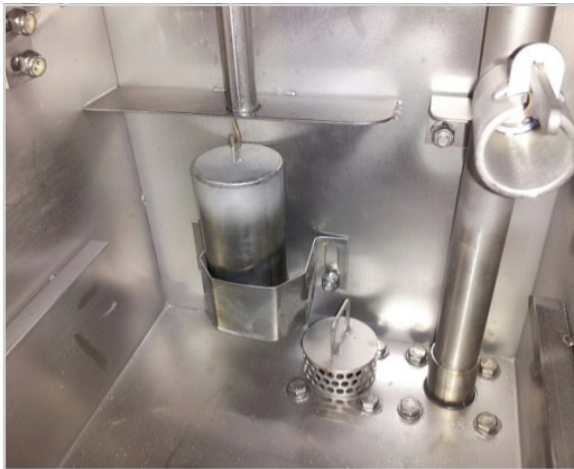
Rinse tank float, pump filter, pumped rinse manifold
