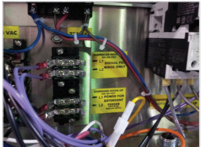
Dispenser signal connection terminals in control box
