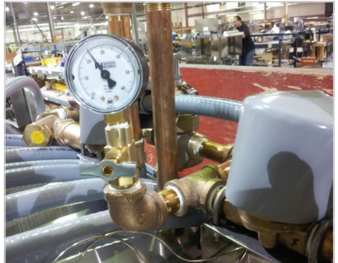
Final rinse manifold with pressure gauge, 20 psi flow req.
