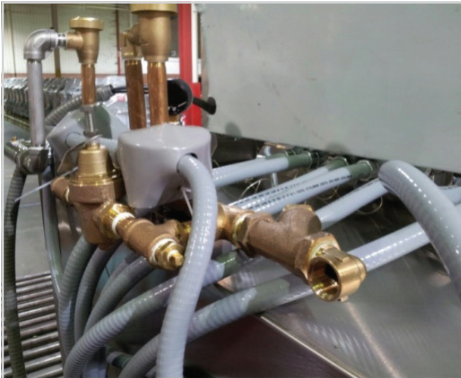
Hot water inlet manifold, single point 3/4" pipe, PR valve
